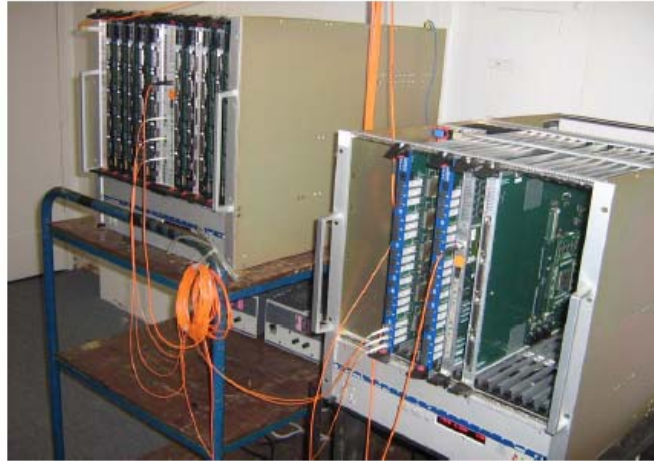
Figure 2: Chain Test in the Peripheral and Track Finder crates
